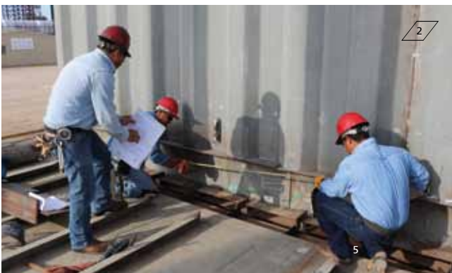
1 The Training Center provides training in areas such as welding and piping work
